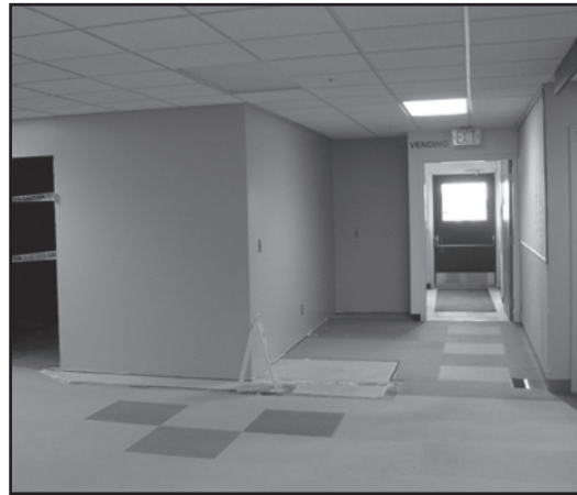
Remodeling begins at Annie Jeffrey Health Center with an anticipated completion date of August 1st.
